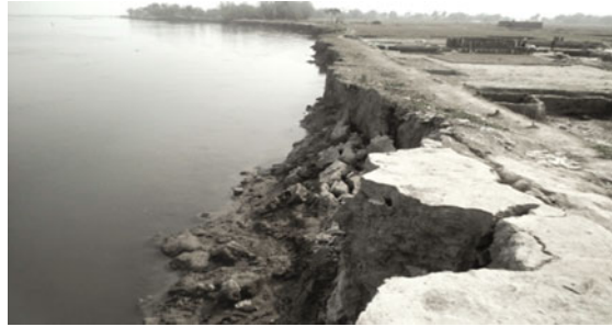
Fig. 2 Eroded river bank at Jiabharali lower plain reach
